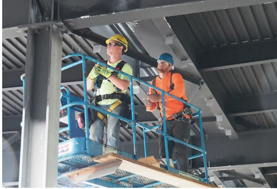
Team members take safety seriously and implement safety standards throughout completion of project.
