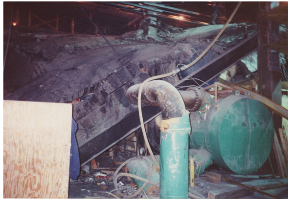
Fire Charred Concrete Floor Slabs and Collapsed Steel Framing Lying on Top of the Refrigeration Equipment (Chillers and Piping) at Bottom of Crater at B-5 Level
