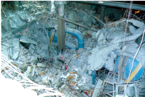
Collapsed Slabs from the B-1 and B-2 Levels Crushed the Refrigeration Plant Equipment on the B-5 Level
