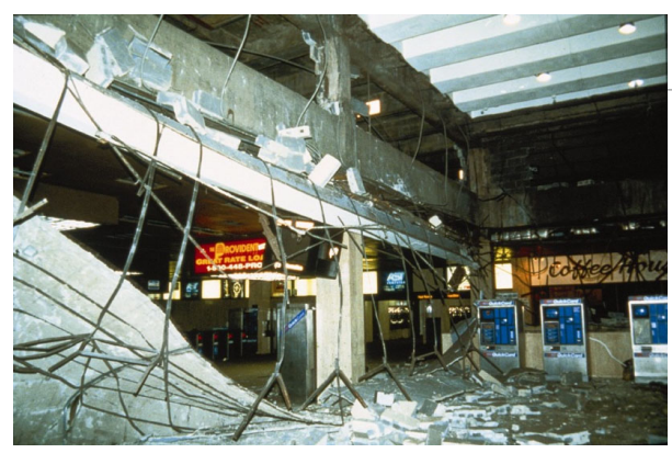
Collapse of Parking Garage Walls & Finishes From B-3 Level Fall onto the PATH Station Fare Collection Zone on B-4 Level
