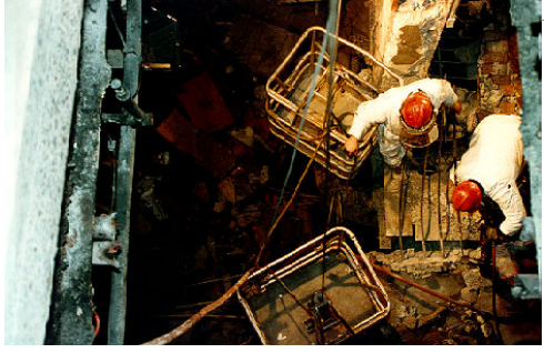
Iron workers entering the subgrade "crater" through an access hole cut through the Vista Hotel Concourse Lobby. They will use Spider Baskets to Install Steel Bracing Members on Unbraced Columns Supporting the Vista Hotel
