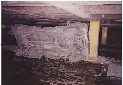
Vehicle at B-2 Level Overturned by Blast Pressure
