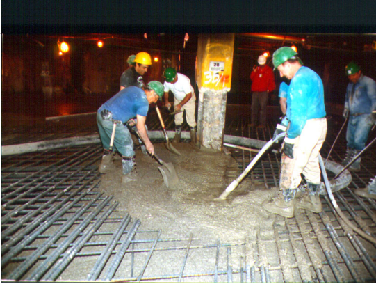
After Placement of Reinforcing Steel on Top of Steel Decking Structural Concrete is Pumped, Cast and Finished
