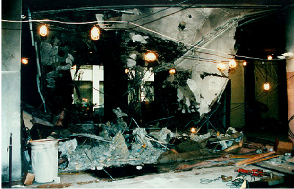
Damage at the WTC Concourse Level (Main Lobby Elevators in 1 WTC Seen in Distance). The Blast Vented Upward Through the Hole in the Floor. (The WTC Plaza Slab Above this Level Buckled Upward but Did Not Breach)
