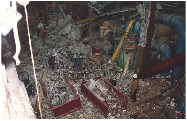
Debris Being Placed in Bins at B-5 Level to be Transported Off-Site for Inspection by FBI and ATF
