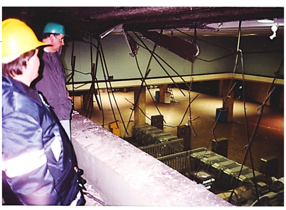
Looking Down on B-4 Level PATH Fare Zone From B-3 Level After Debris Clean Up. PATH System was Found to be Operable.
