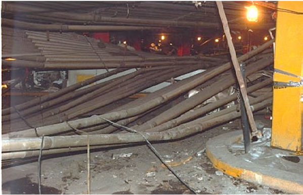
Collapse of Utilities from Blast at B-2 Level NY Telephone Company major telephone exchange at the WTC complex providing telephone service to Lower Manhattan also providing service for air traffic control systems at the three major NY-NJ airports
