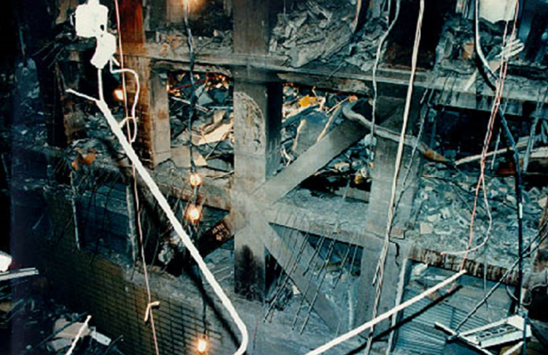
B-2 Level Damaged Tower Column and Missing Bracing Member
