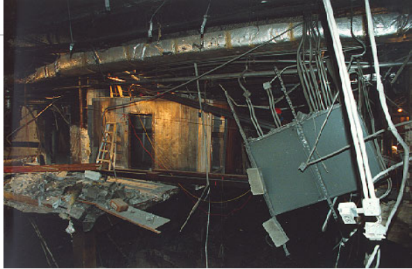
Damage at the B-1 Level Where the Was a Large Section of Floor Slab that Collapsed Adjacent to the Operations and Control Center
