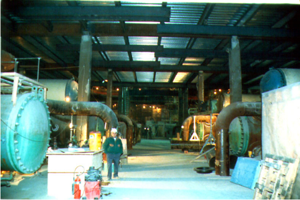
With Steel Decking In Place Work on Repairing the Refrigeration Plant Could safely Proceed
