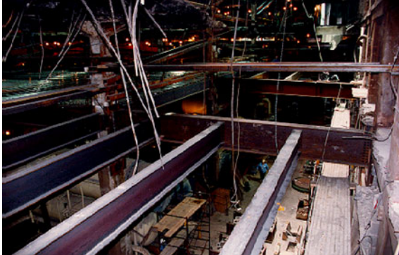
Steel Framing Being Installed to Replace the Collapsed B-2 Level Floor system That Spans Over the Refrigeration Plant
