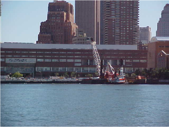
September 16, 2001 (Day 5): Dredging south of Pier 25, near bulkhead, for preparation of transfer site for debris removal to Fresh Kills Landfill, Staten Island, NYC.
