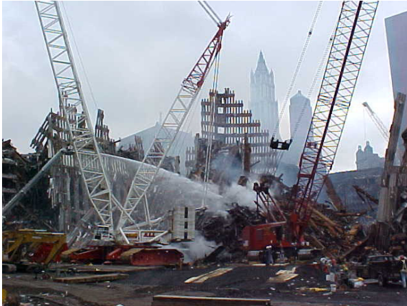
Sept 26, 2001 (Day 15): Tower 1 still burning. Sub-basement 6 flooded. Temperature at sub-basement 5 measured at 1,200 degrees F. Sub-basements 4, 3, 2, & 1 collapsed. Site is changing from recovery to a demolition project.
