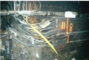
Deteriorated Duct Bank Cables at Splice Chamber
