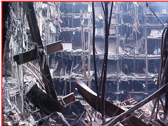
Core of Damaged Building
