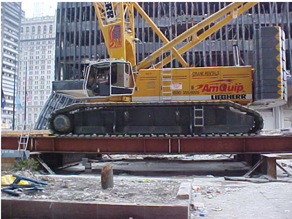
Sept 20, 2001 (Day 9) : Grillage was placed to support 310-ton crane, placed above concourse level, between Bldgs. 4 & 5. Northeast Plaza Building (Bldg. 5) in background.
